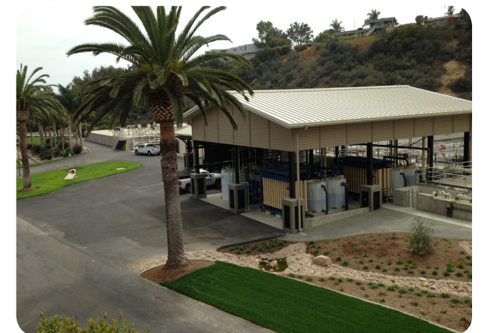
Recent construction of advanced water treatment facilities at the San Elijo Water Reclamation Facility allows for increased recycled water production using high-salinity influent.
